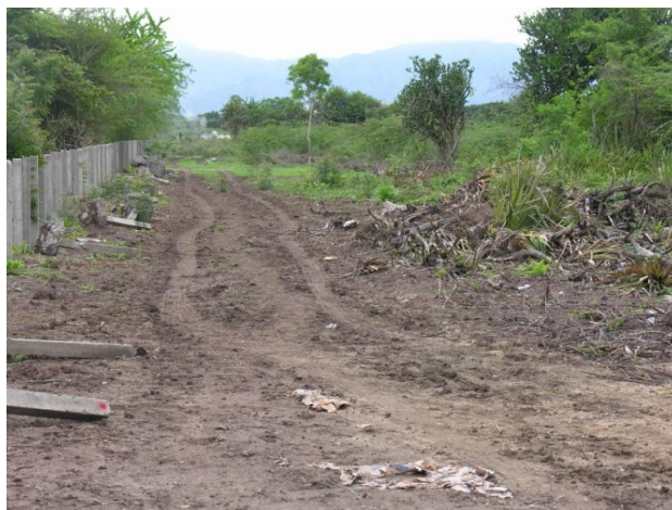
Photo 19. Clearing to provide an access road to the location of the future power plant has already begun
